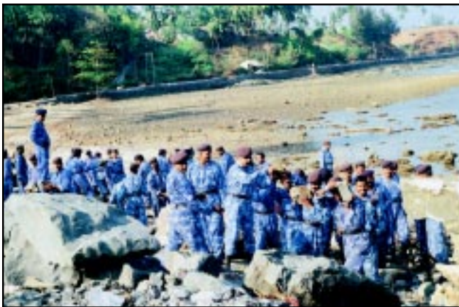
99 RAF personnel repairing Culvert Road near sea, South Point, Port Blair (A & N), India
