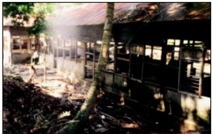
Destruction caused by Tsunami in Nancowry
